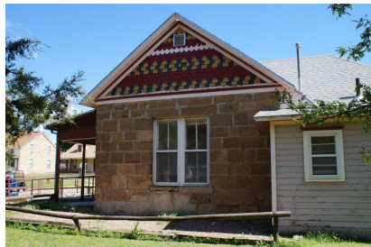
Fort Dodge - Officers House. 702 Sheridan Street. South elevation of original building (left) and wood-frame addition (right); looking north. 05/25/2017. KSHS/Anderson, Rick.
