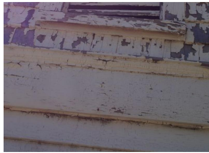
Fort Dodge – Dead House (Relocated). 317 Pershing Street. North elevation louver; looking south. 08/16/2017. KSHS/Anderson, Rick.
