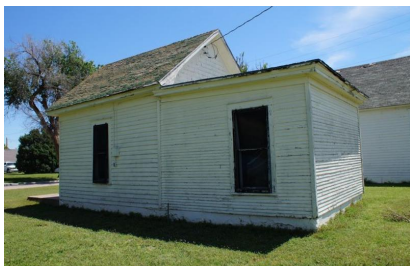
Fort Dodge - Dead House (Relocated). 317 Pershing Street. West elevation of the original building (left) and shed addition (right); looking north-northeast. 05/25/2017. KSHS/Anderson, Rick.
